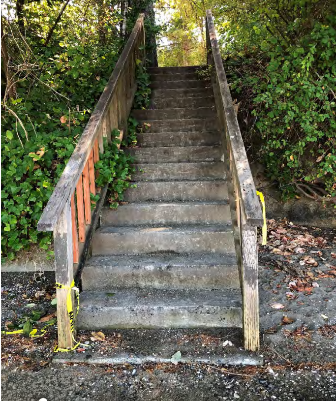
Photograph #-12. Western Beach Access Staircase (Concrete with Wood Railing), Natural Shoreline to Right
