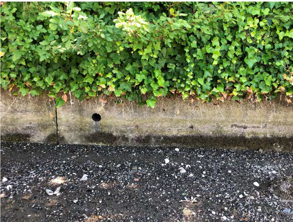
Photograph #8. Toe of Concrete Bulkhead to the West of the Eastern Access Staircase
